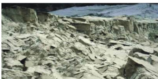
Figure 5. Upstream slope deformations of retaining dyke caused by settling of underlying slimes
